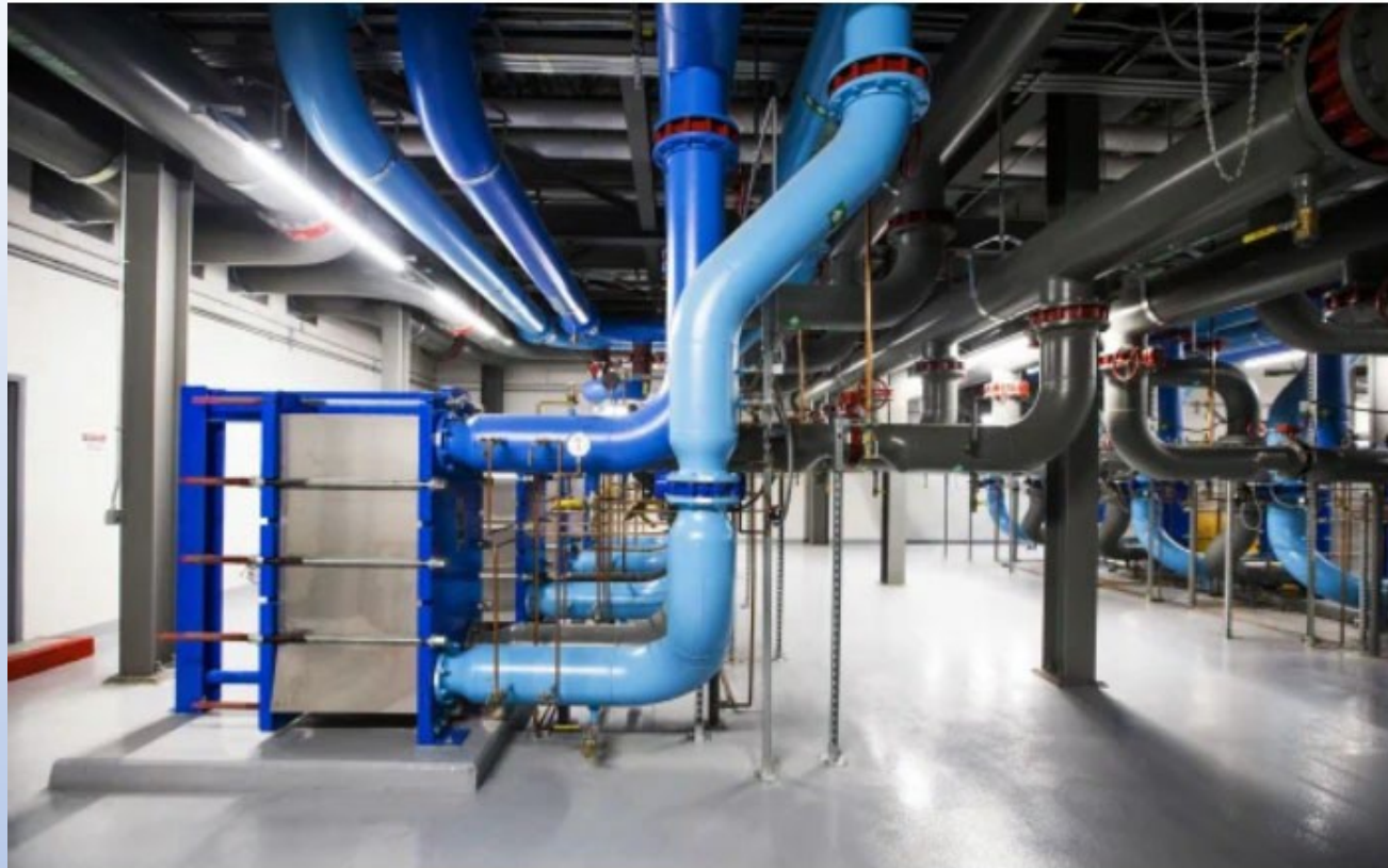
— The system used to cool servers inside the Apple Data Center in Mesa, Ariz.
